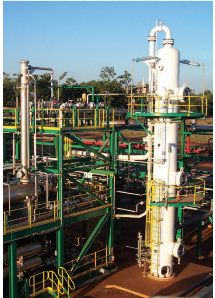
ENI Blacktip Gas Processing facility Location: Northern Territory, Australia
