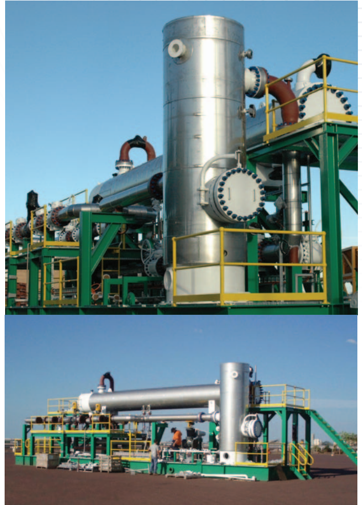
ENI Blacktip Gas Processing Facility MEG DPCU package Location: Northern Territory, Australia
