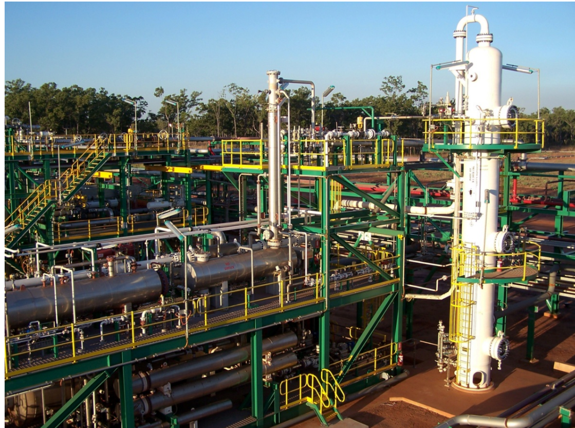
ENI Blacktip TEG Dehydration package installed at site, Northern Territory 2009.
