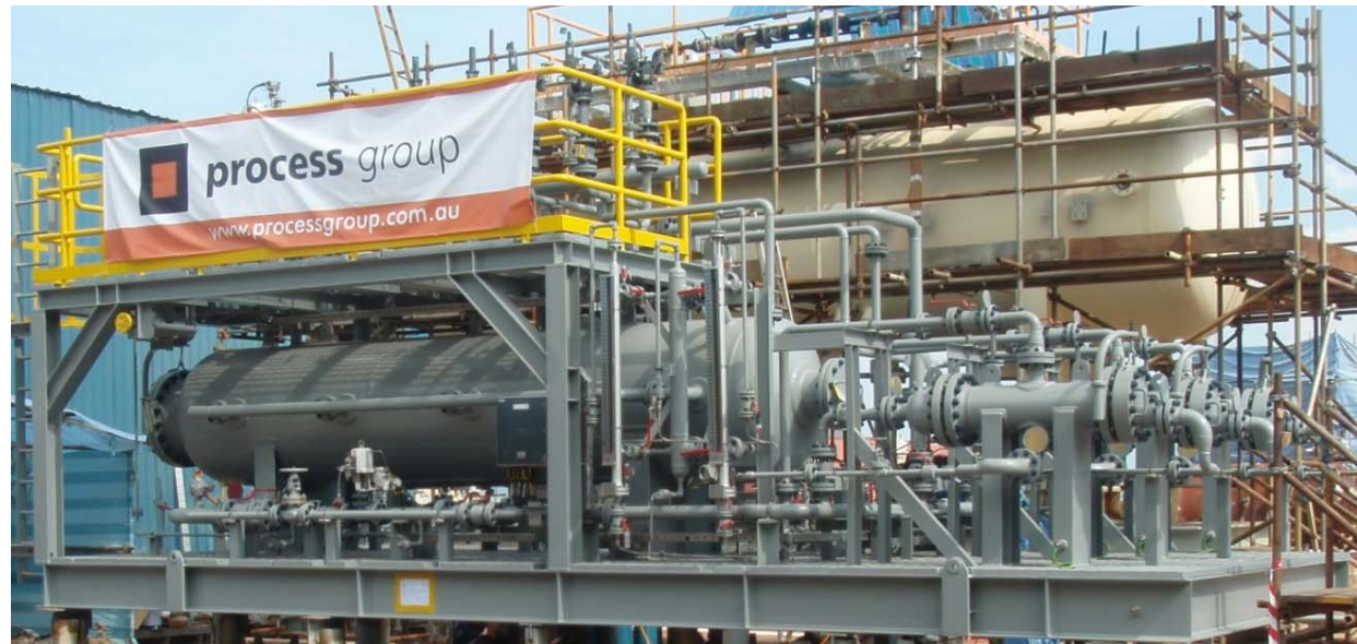
Three (3) Deoiler Hydrocyclones on the right feeding into a single Dissolved Gas Flotation Unit
