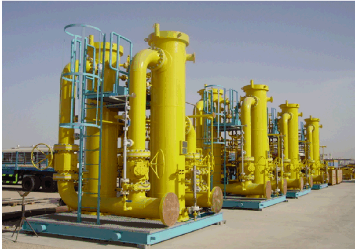
Inlet Scrubber Vessels of the Gas Pressure Reduction Stations ready for delivery at Process Group International's workshop, 2006.
