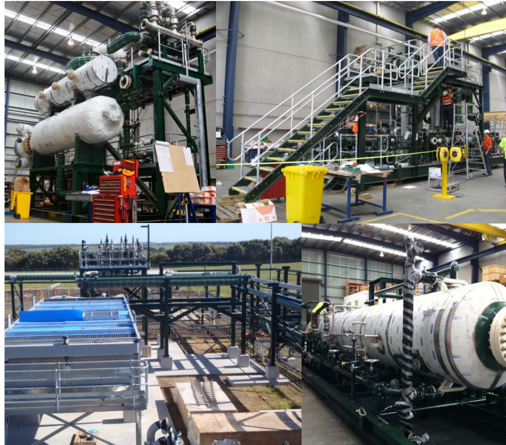
Refrigeration package and gas chiller skids under construction at Process Group's works and being installed at site, 2011.
