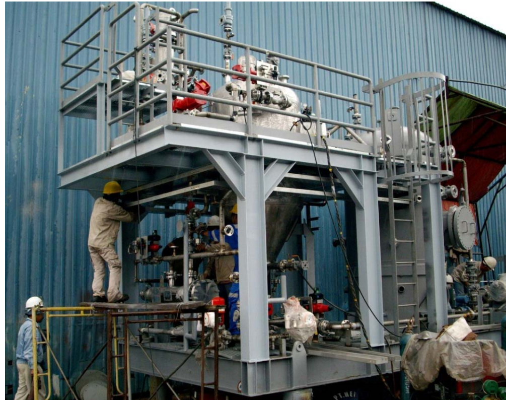
Sand Handling and Cleaning Package for WHP-D nearing completion at Batam works, Indonesia 2007.
