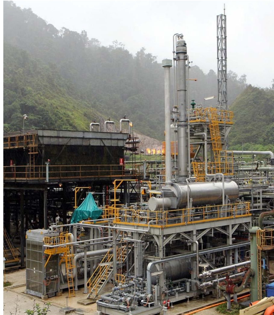
Installed TEG Dehydration package, Papua New Guinea.
