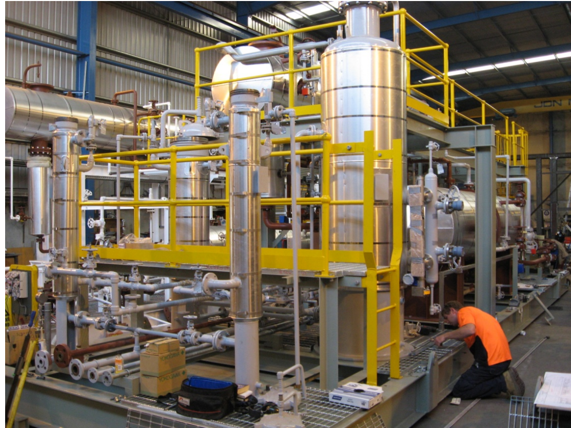
Strathblane TEG Regeneration skid being prepared for delivery at Process Group's works, Bayswater 2008.
