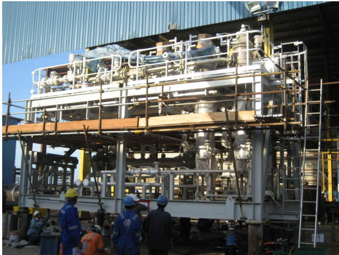
Fuel Gas package being prepared for delivery, Batam works.
