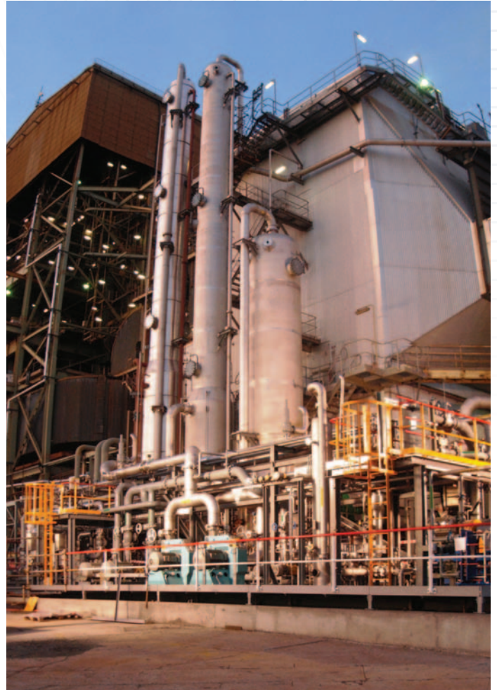
Hazelwood Power Station Carbon Capture Plant Location: Victoria, Australia
